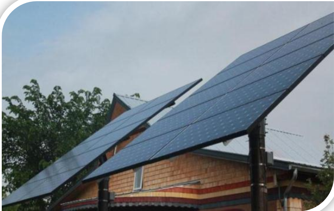
Solar panels at the Camp Kawartha Environment Centre.
